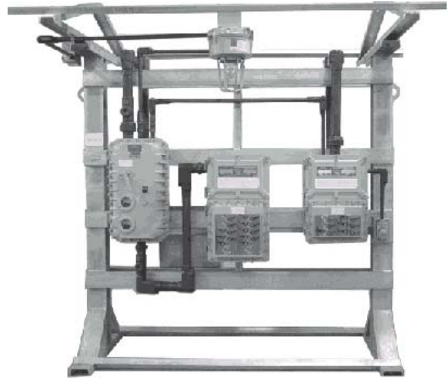
Switchracks may be single or double sided, with components mounted in single or double rows.
